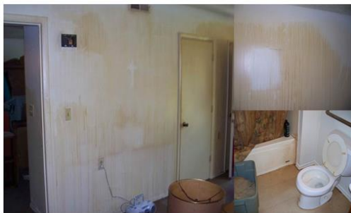
Damage to an apartment in Brunswick County after 7 years of heavy smoking. Photos courtesy of Ernest Watts, NC TPCB Region 8 Manager
